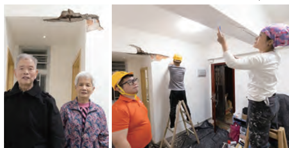
Under the Home Repair Services Community Programme, URA arranges building inspection and minor structural works to enhance the living conditions of elderly individuals (left) residing in old buildings.
